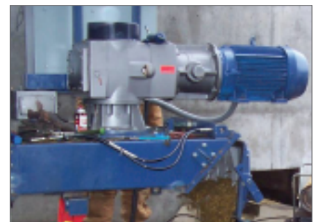
Main Drive Gear Box and Motor
